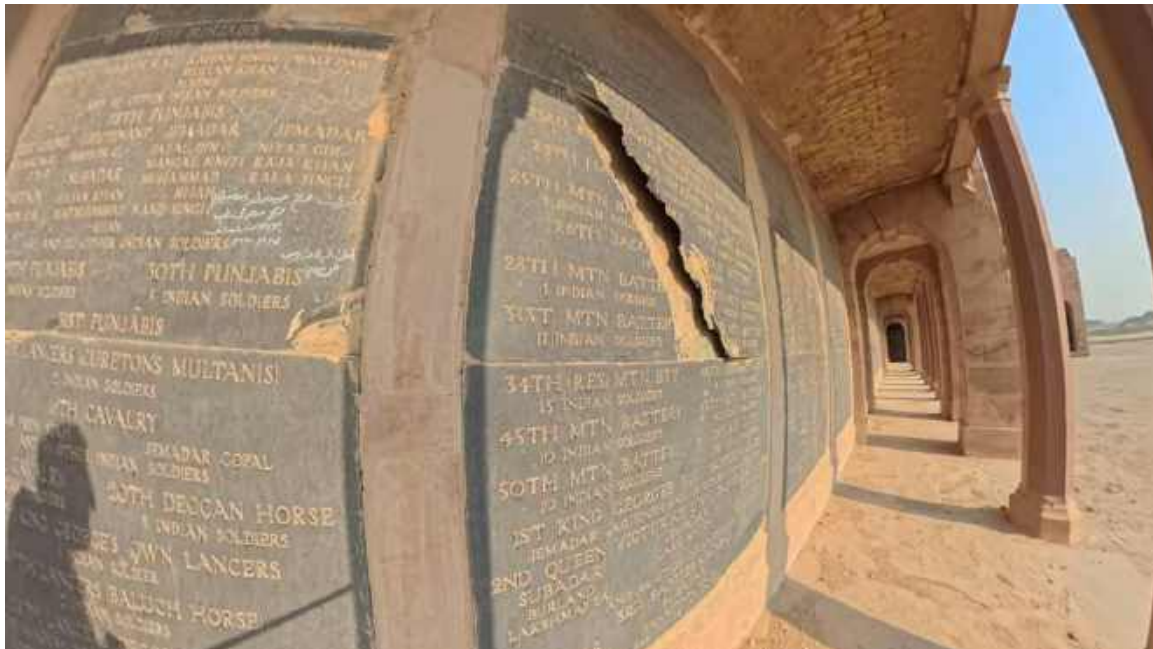
Panel 46 Nov 2025 delamination
